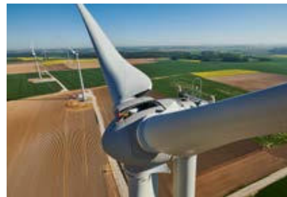
Coquelicot wind farm, France. Photo: Jan Oelker
