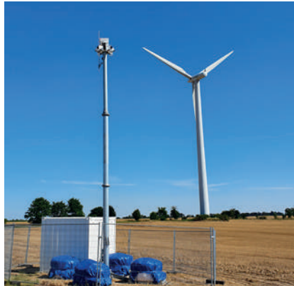
Stand-alone installation of IdentiFlight.
