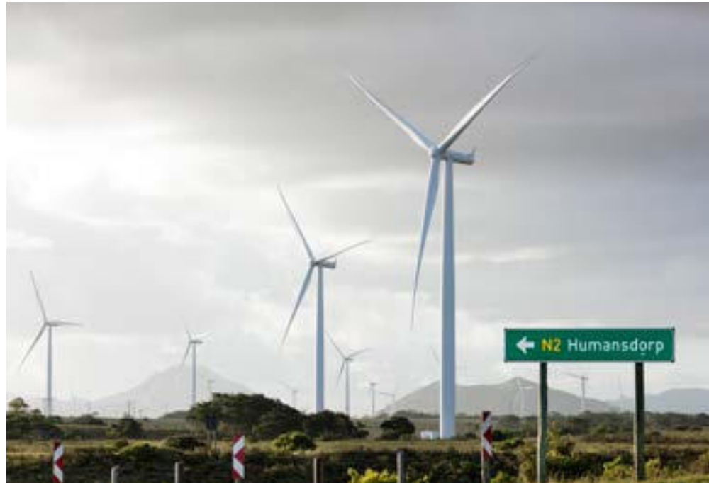
Jeffreys Bay wind farm, South Africa, with 60 SiemensGamesa wind turbines. Photo: Paul-Langrock.de
