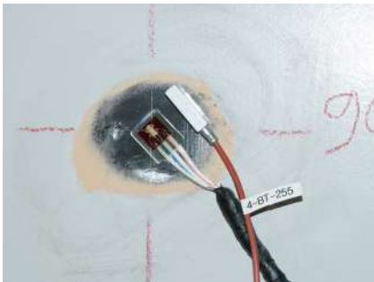
Recording the stresses of the steel tower by measuring the strains using strain gauges
