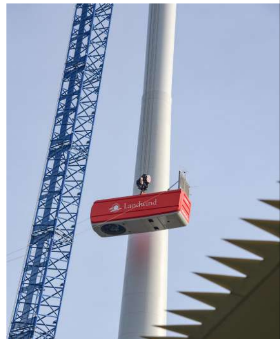
Machine house assembly
