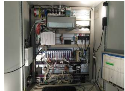
Central measuring station at tower base for recording and transmitting of all monitoring data
